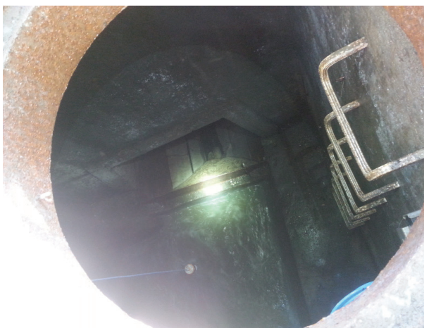
A sample installation of a SmartWeir™ in a CSS regulating structure. The ultrasonic sensor is hanging from the ceiling of the structure in the lower part of the photo, and the overflow weir is above, where the light is shining.
